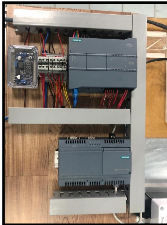
Figure 4: PLC that used in the project
